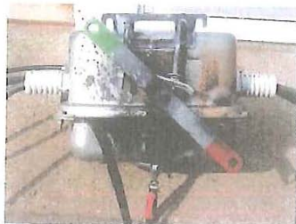
[高圧区分開閉器側面]
