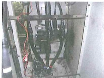
[真空遮断器裏側]
